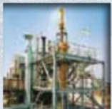
Waste gas scrubbing plants
